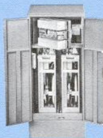
Rear View of cabinet shows doors and hinged relay rack.
